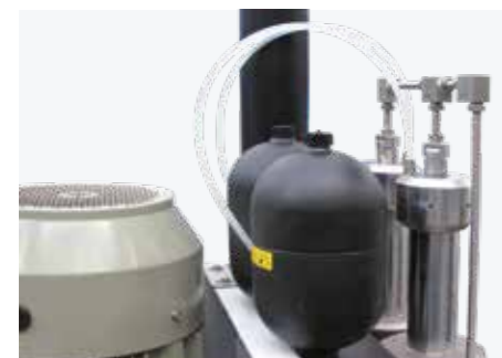
Nitrogen accumulator for managing the hydraulic cylinders return circuit
